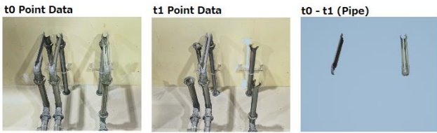
Fig. 6 Differential extraction example 2: pipes removed Shape recognition (semantic segmentation) using deep learning is then performed on the extracted differences, such as those shown in Figs. 5 and 6. In the examples, shape recognition is performed for the added shielding plates and the removed piping (Fig. 7).
